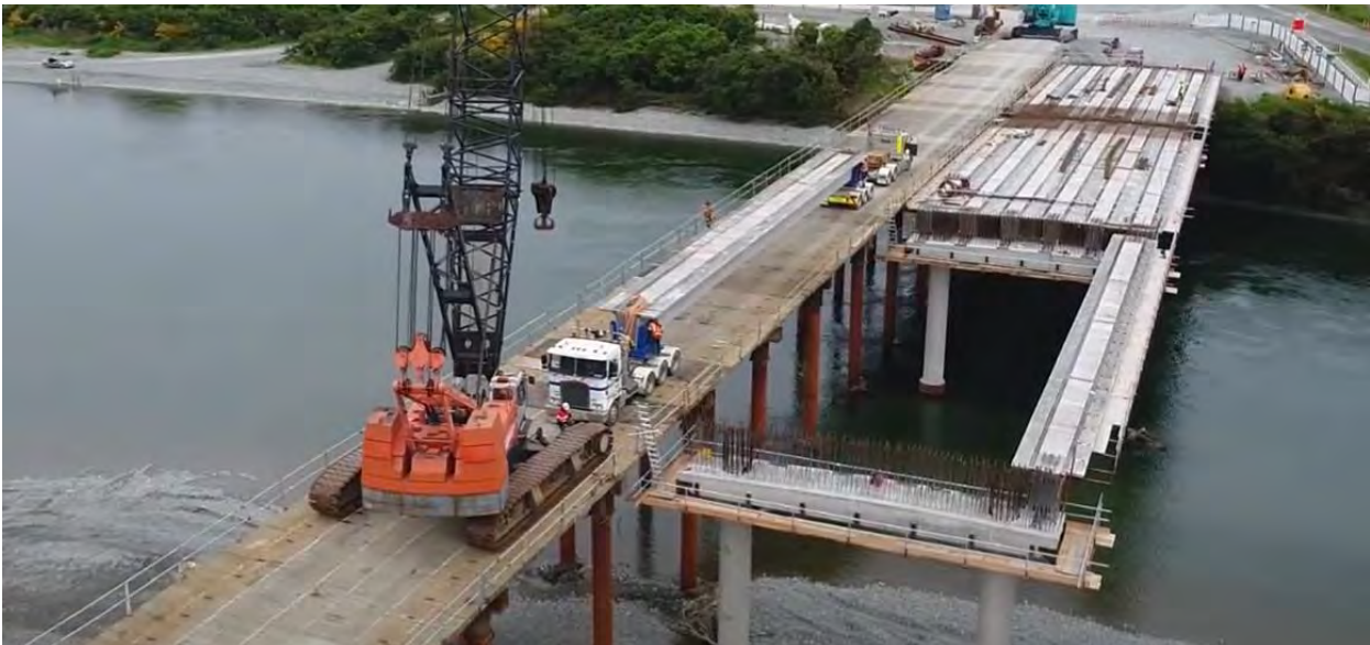
Figure 4 - Typical temporary staging – the orange crane and truck are sitting on the temporary staging. The new bridge is to the right
